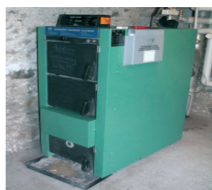
Central heating furnaces
